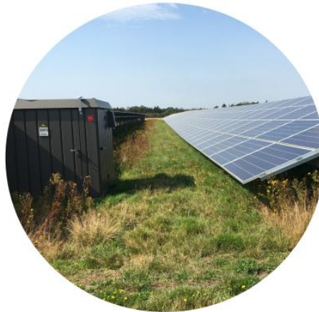
Transformerstation imellem solcellerne
