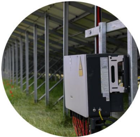
Inverter - placeres bag/under solcellerne
