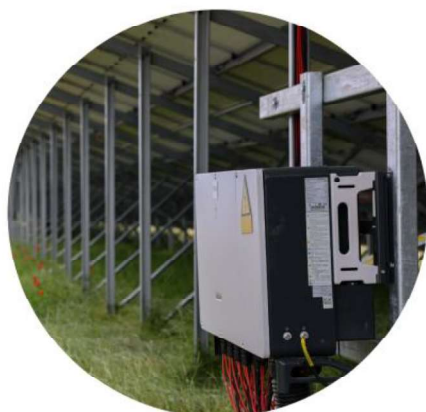
Inverter - placeres bag/under solcellerne
